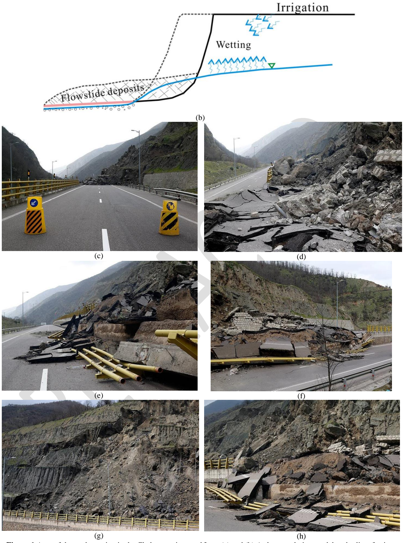
Figure 1 Area of the study section in the Chalus province and Iran: (a) and (b) A slope evolution model under liquefaction condition; (c), (d), (e), (f), (g) and (h) landslide caused by soil liquefaction
