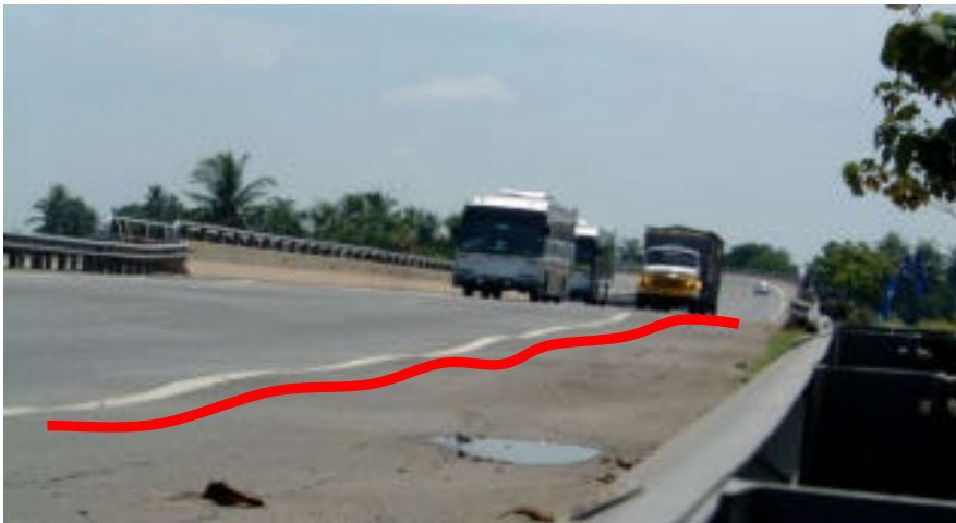
Figure 8 “Mushroom” Undulating surface on an expressway (Modified after [9])
