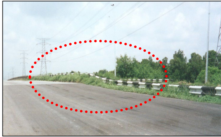
Figure 5 Hump at bridge approach
