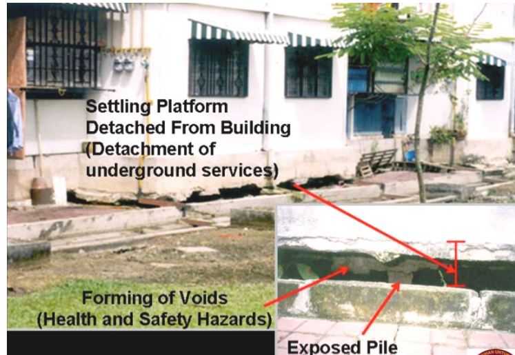
Figure 2 Settlement of platform over soft ground and detachment from building with piled foundation
