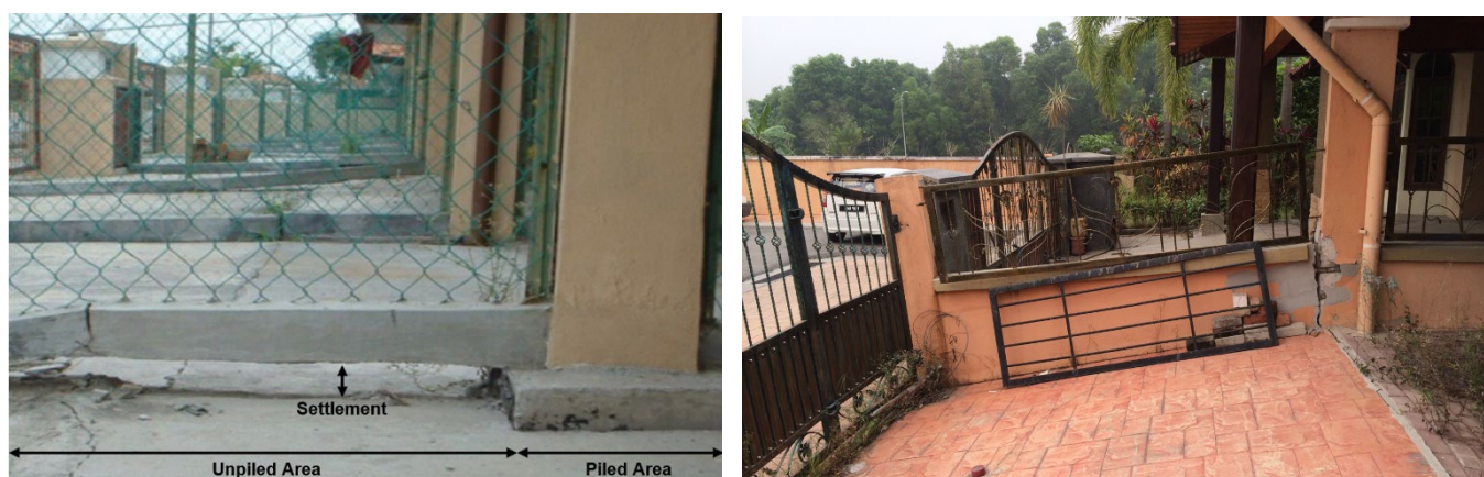
Figure 1 Examples of differential settlement of piled and unpiled area.
