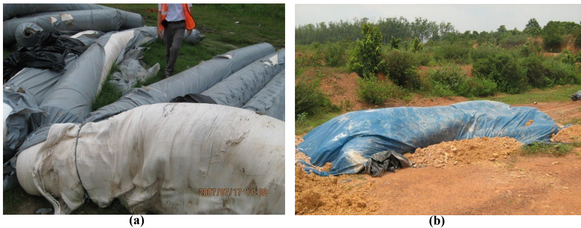
Figure 15 Improper (a) and proper (b) storage of geotextile at site (Modified after [18]).
