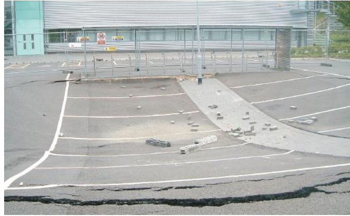
Figure 2 Failure of geocellular tanks after three years [2]
