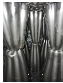
(c) Misplaced of the column interlocking
