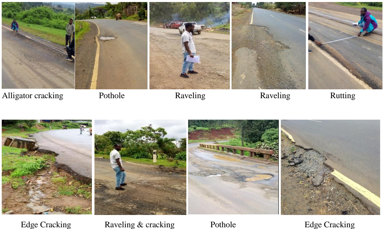
Figure 2 Pavement failure types were observed along the road segment.
