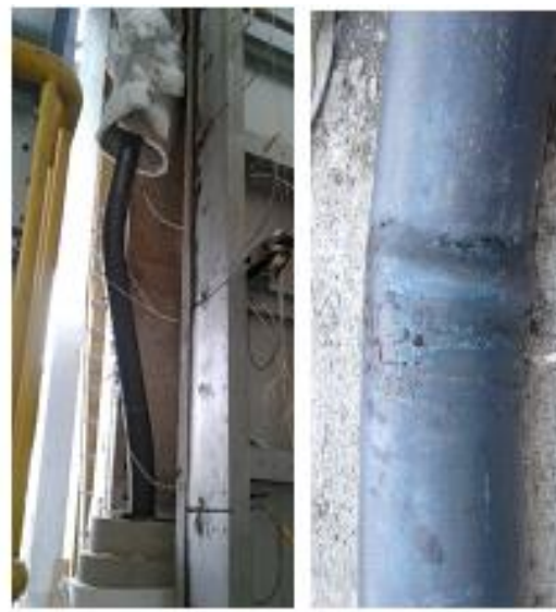
Figure 4: Failed foamed concrete filled column
