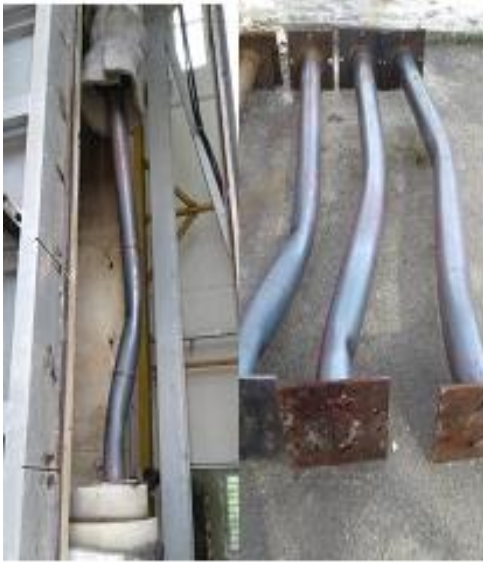
Figure 3: Failed unfilled hollow column
