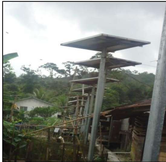
Figure 3. Existing Solar Panel.
